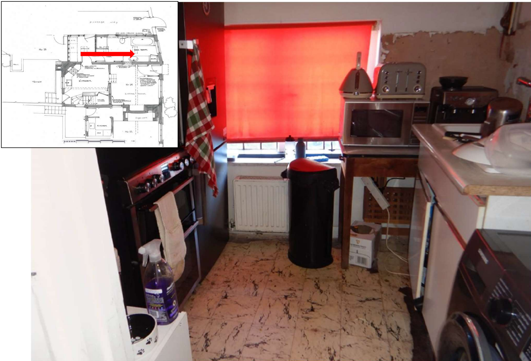
Figure 2: Existing kitchen into the lean-to area that is proposed to from the new bathroom with new gas boiler in the far right-hand corner of this photograph with flue through the monopitched roof.
