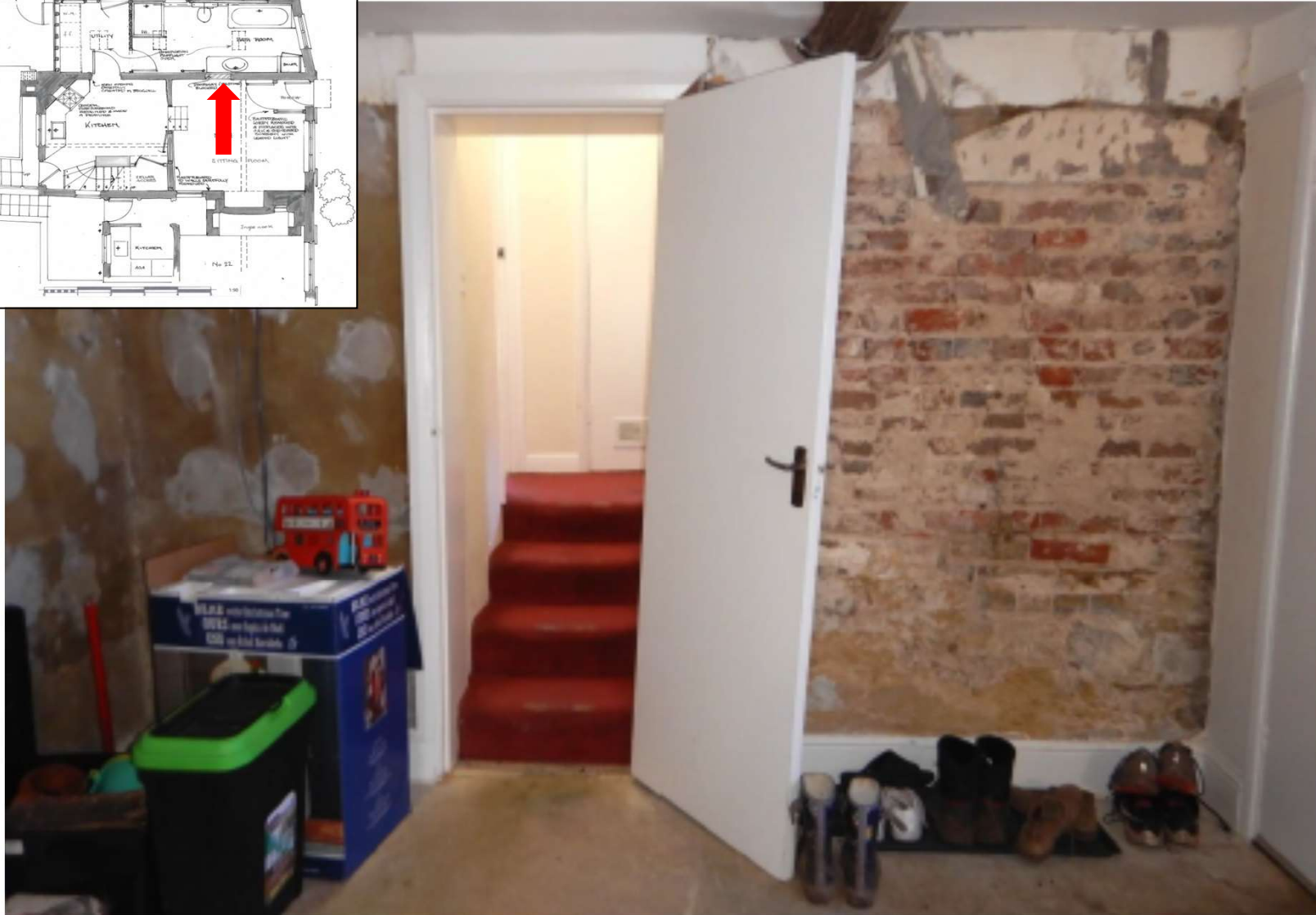
Figure 1: Steps to bathroom and kitchen currently located in the lean-to (to be blocked up)
