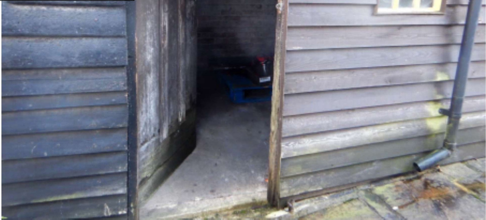
Figure 8: Doorway from the passageway into the proposed utility area. External featheredged weatherboarding to be retained where possible and thermal insulation added internally
